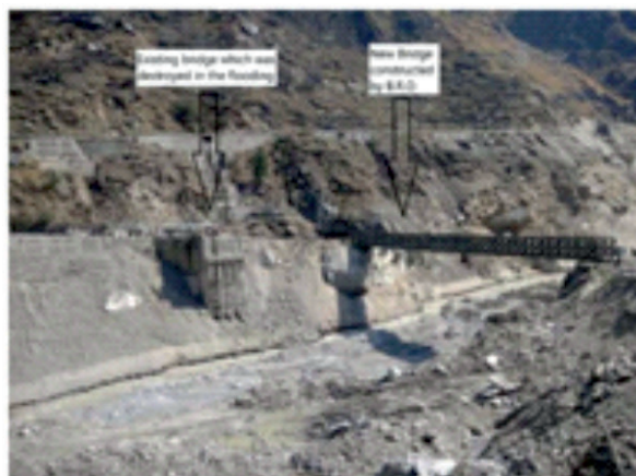
Fig - 51 : Remnants of damage BRO motor bridge withbailey bridge constructed by BRO for vehicular movement on Joshimath – Malari road after the event
